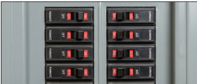
PUSHMATIC / BULLDOG — push-BUTTON breakers, no toggle handles
